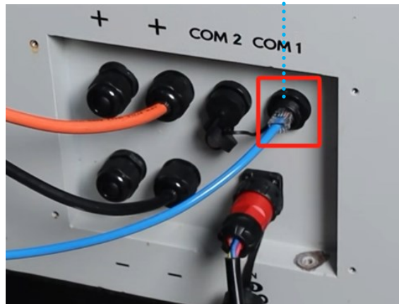
Pic 1.1.2 HV48100 SE COM1 port (outside of cabinet)
